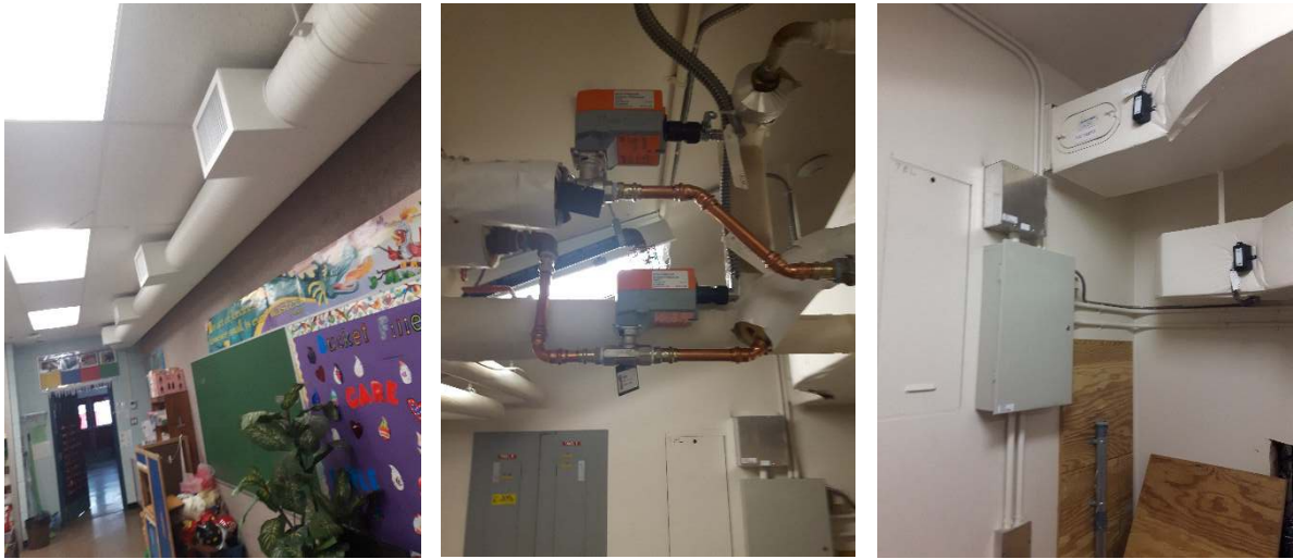
Figure 5 - Royston Elementary School HVAC (Mechanical) & DDC Replacement
