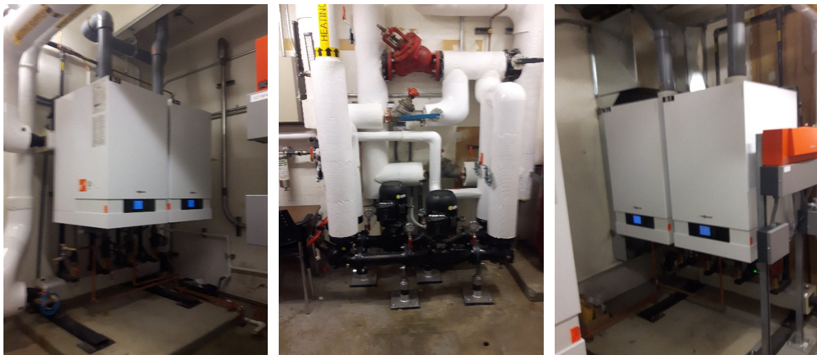
Figure 7 – Ecole Puntledge Park Boiler Plant Upgrade Project: four new high efficiency Viessmann condensing boilers and pumps.
