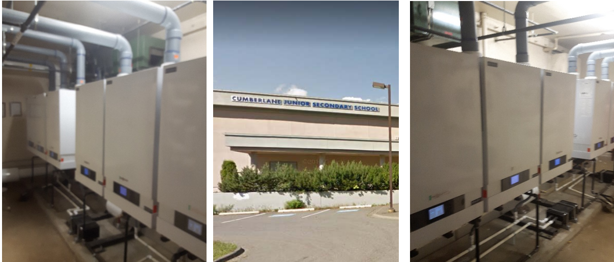
Figure 5 – Cumberland Community School Boilers (pumps also replaced).
