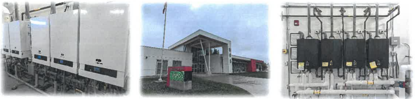
Figure 4 – New Viessman boilers, Lake Trail Community School entrance & on-demand hot water heaters
