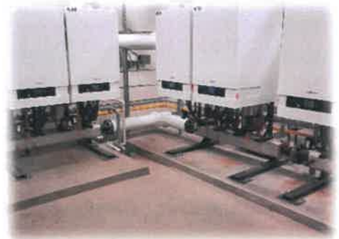
Figure 2 – New boilers installed at Aspen Elementary
