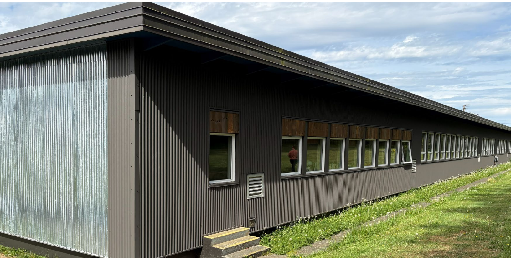
North Island Distance Education School – new windows & cladding system on the east side of building (Phase II of the Building Envelope Upgrade)
